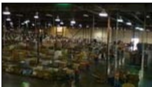
The warehouse had large, inefficient metal halide lights.
